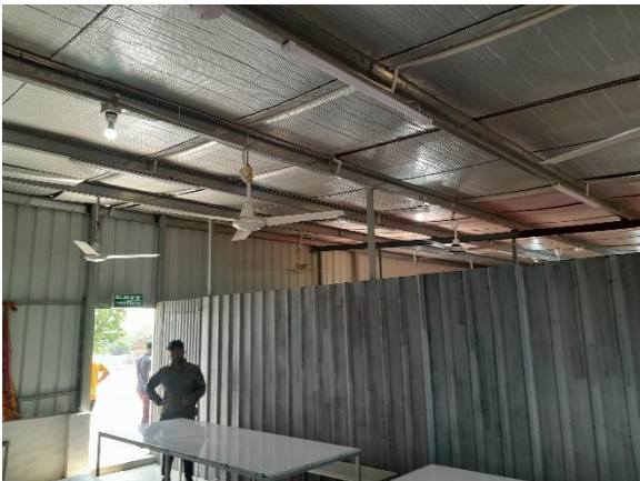
Inadequate members (Roof top shed)
