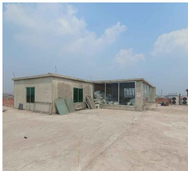
Undocumented extension at roof
