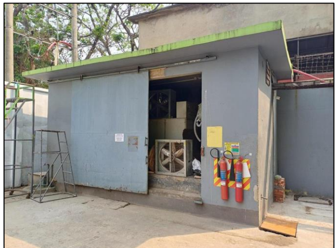
Old Transformer Room
