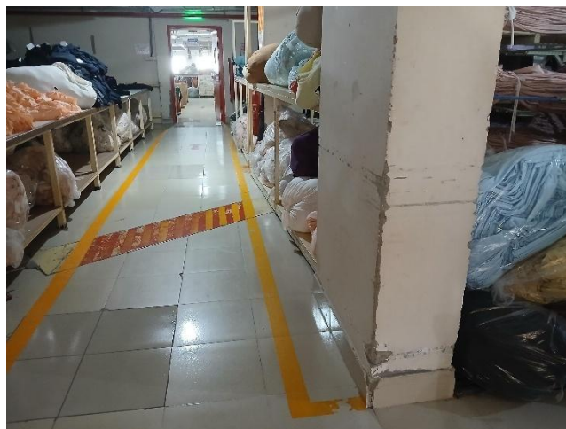
Trolley impact and surface damage on columns
