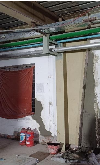
Mezzanine steel column C3 found tapered instead of regular straight shape
