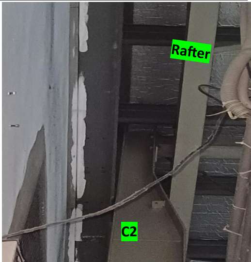
End grid rafter was not rested on column C2, no details found. Also, reduced section size was observed at the top level.
