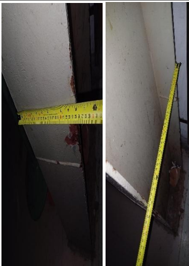
Steel column C2 size found F-255 X W-365 instead of F-300 X W-320
