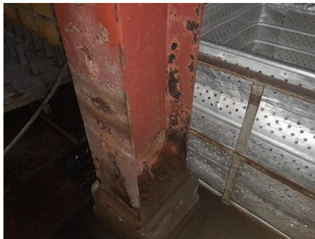
Corrosion on steel member
