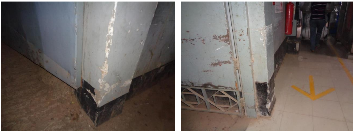
Trolley impact and surface damage on columns
