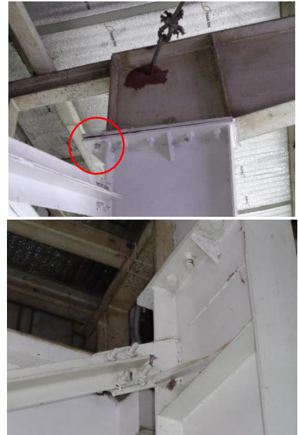
Bolt missing & inadequate edge clearance
