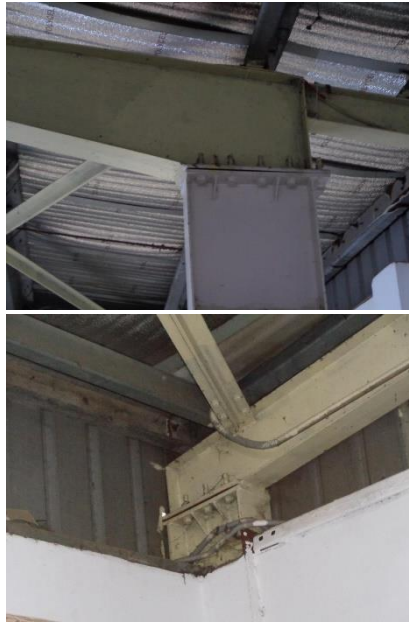
Gap between joint plates
