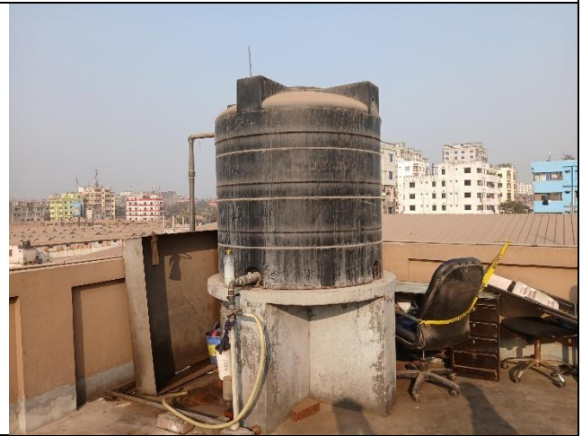
PVC water tank on roof and Open to sky
