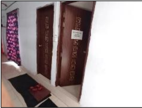
200 mm build-up at 3rd-floor toilet
