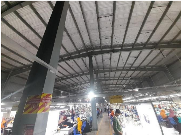
Absence of load transfer media
