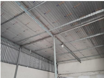
Connection details and rafter layout not matched (Chemical & Wastage Shed)
