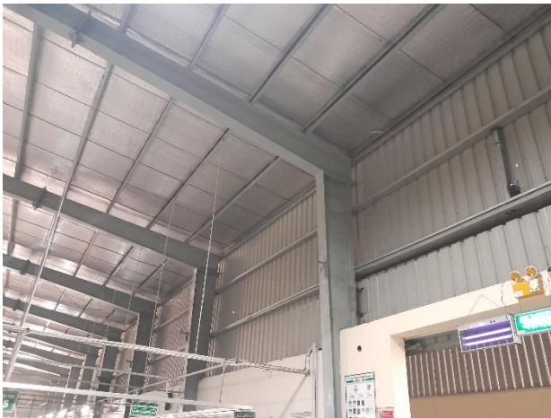
Absence of load transfer media
