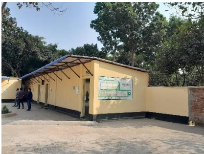
Member size and rafter layout not matched (Office Shed)
