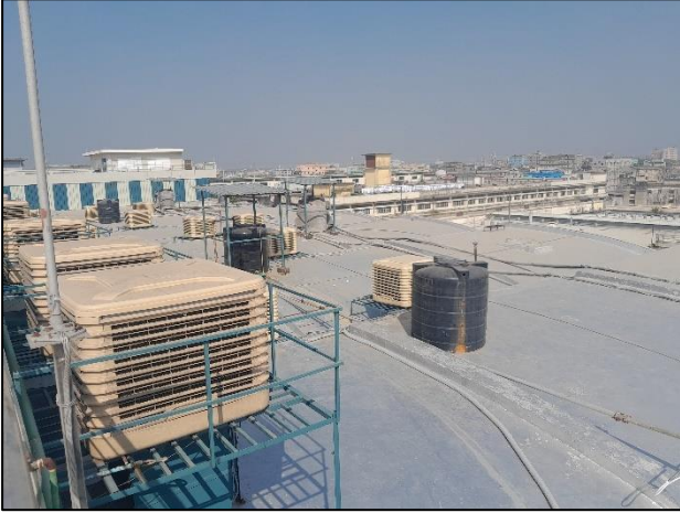
Undocumented plastic water tank at roof.
