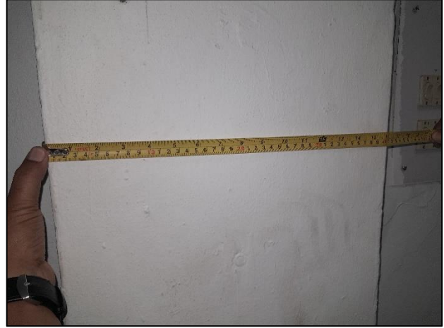
C4 column found 400x400 instead of 500x500 on the ground floor.
