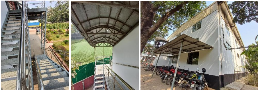
Building 13: lack of lateral stability in Steel stair & parking
