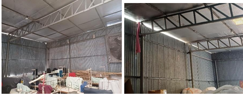
Building 12: lack of bracing & strut in E-W direction.
