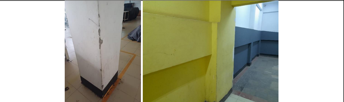
Columns are susceptible to impact
