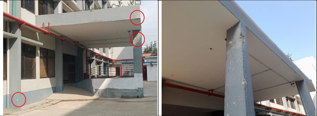
RC columns at the loading-unloading zone susceptible to vehicle impact
