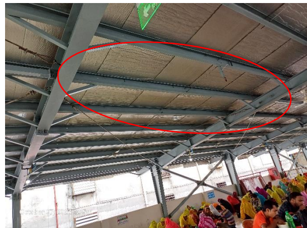
Strut member missing on-site
