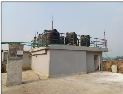
PVC WT on stair roof
