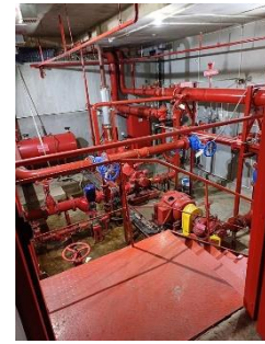
Fire pump at basement
