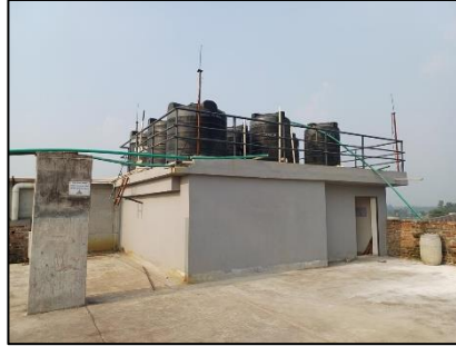
PVC water tank on stair roof
