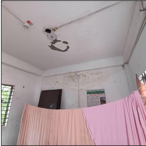
Dampness on roof slab
