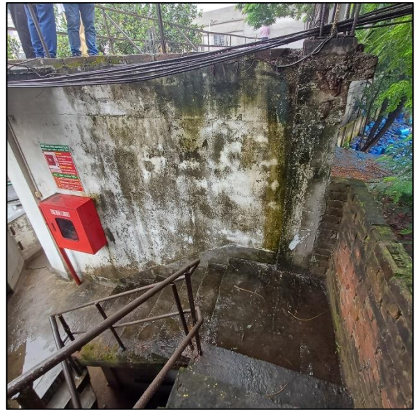
Dampness on wall
