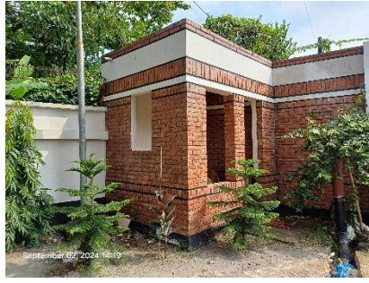
Fire control room
