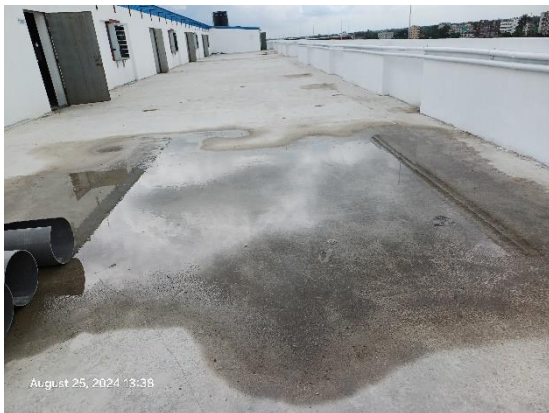
Standing water on the roof level
