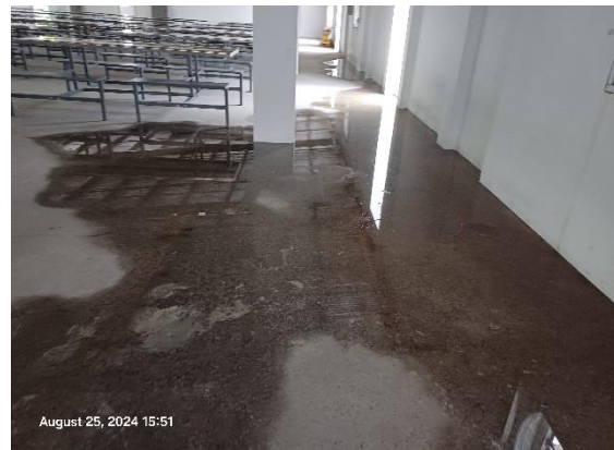
Standing water on the floor of the Dining
