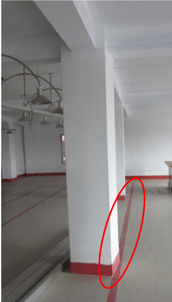
Column was twisted on 5 th floor
