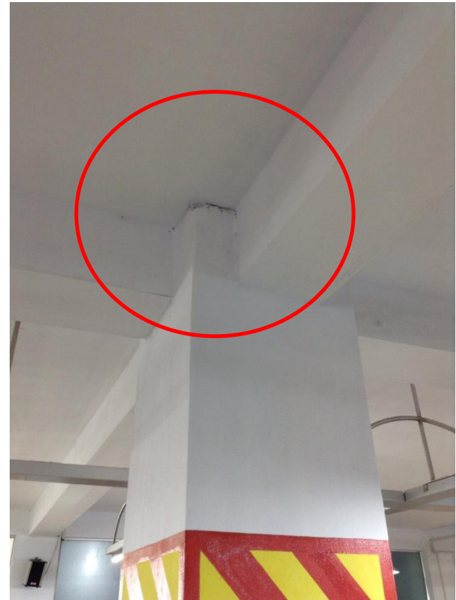
Gap was found between column and slab
