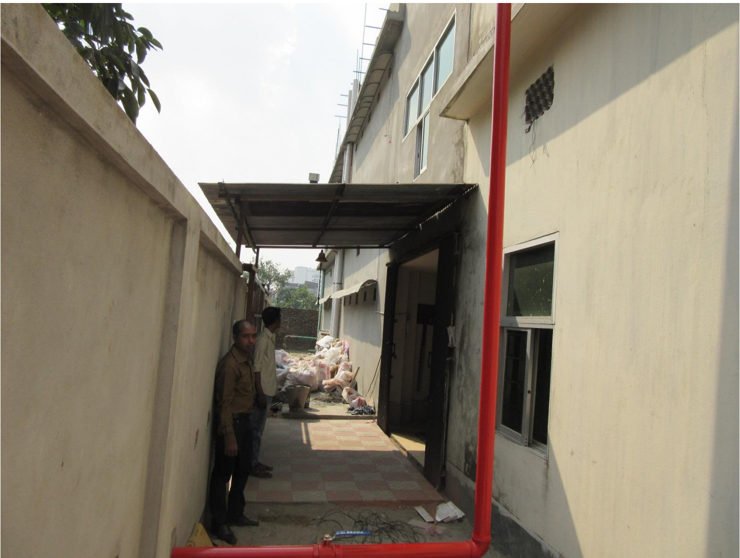
Non-Engineered roof structure attached to the building in an ad-hoc manner.
