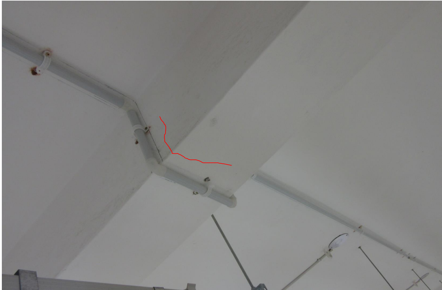
Cracks in some beams in 1 st floor
