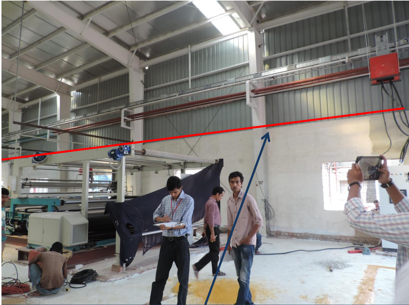
Lack of head restraint to masonry infill wall panels
