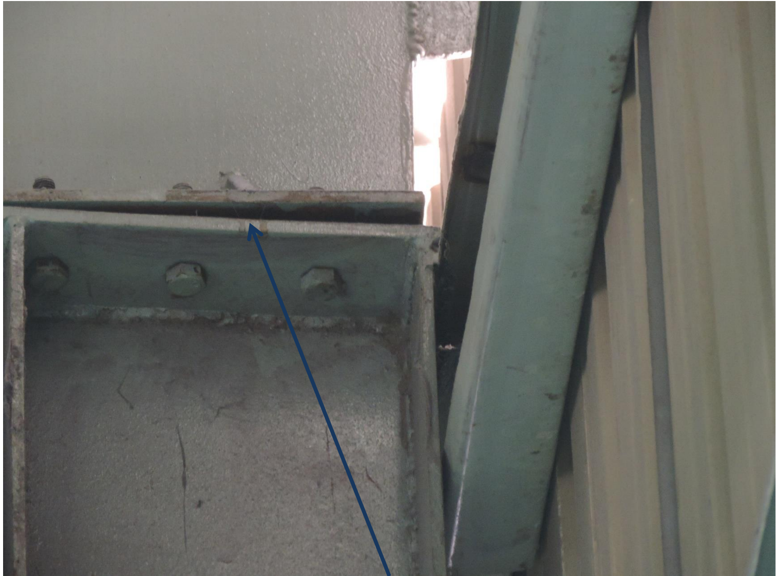
Open moment joint in portal 10
