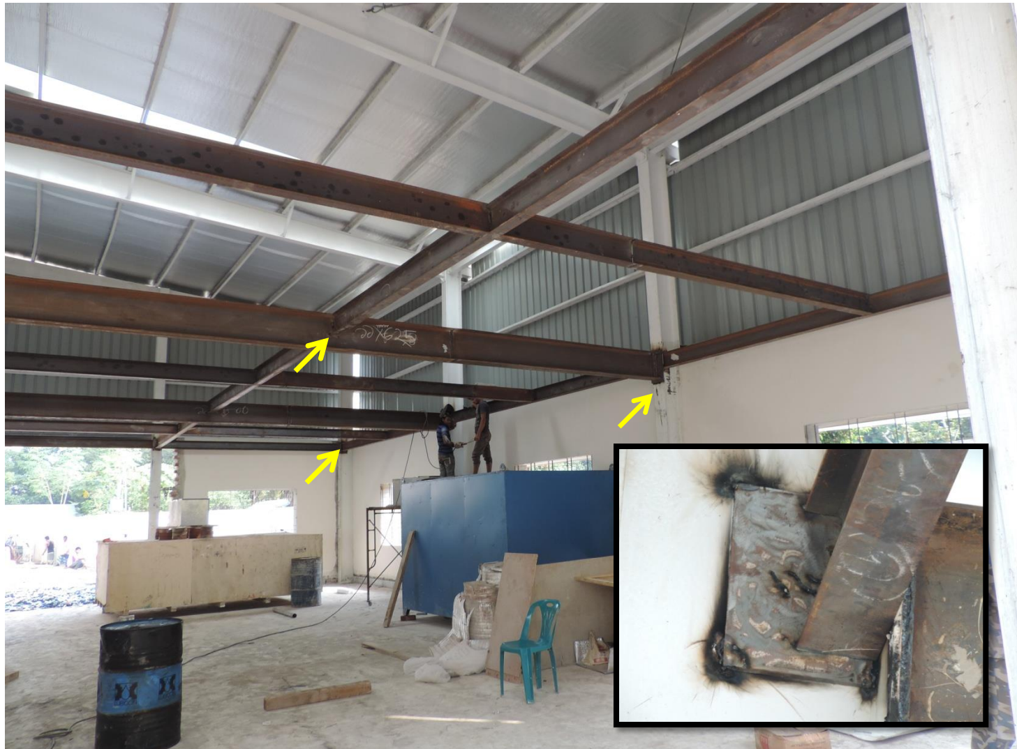
Non engineered connections to mezzanine floor. On site welding
