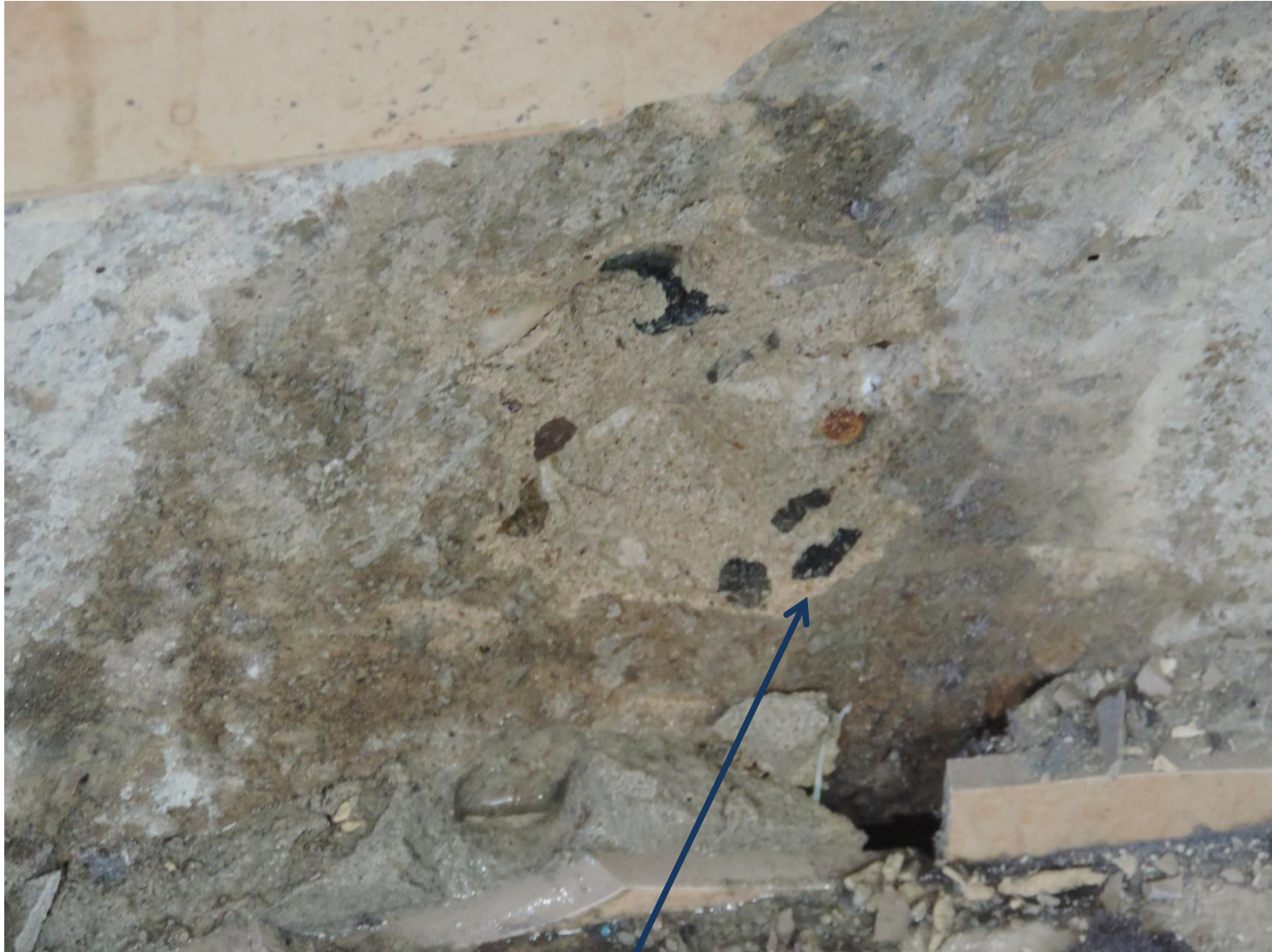
Stone chips observed at ground floor column
