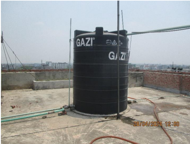
Unbraced water tanks on roof
