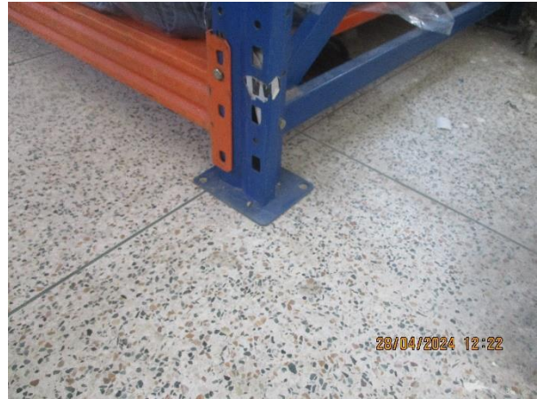
Unbraced racks on the floor
