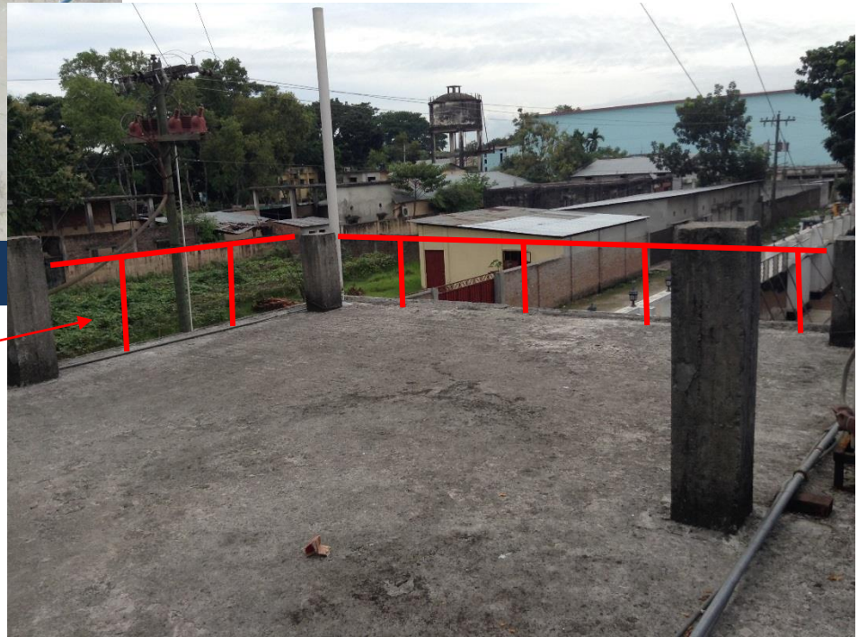
Lack of parapets or fall restraints
