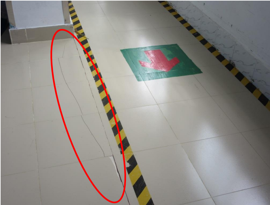
Cracks on the ground floor – internal, South.
