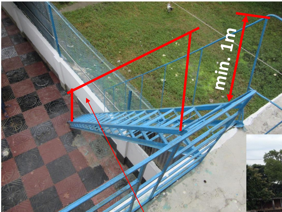
Lack of hand rails
