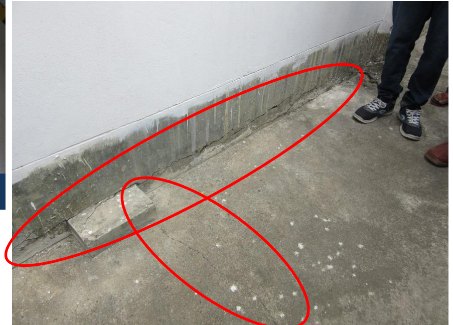
Cracks on the pavement – external, South.
