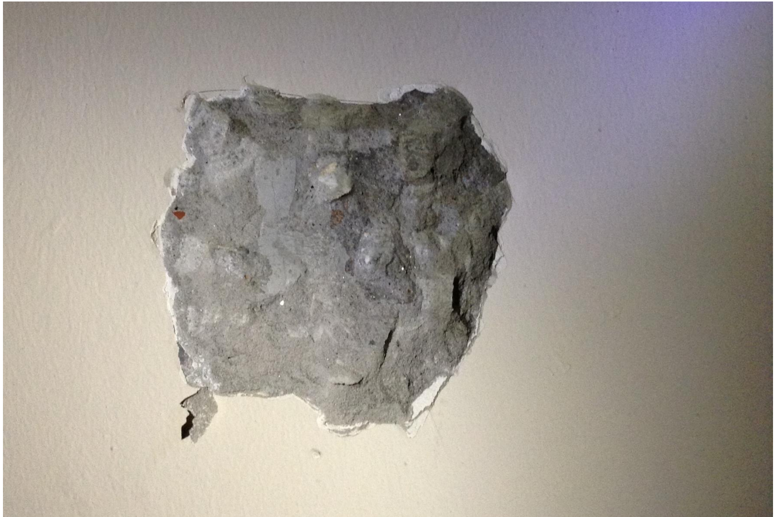
Stone chips observed in column
