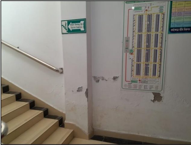
Dampness on wall
