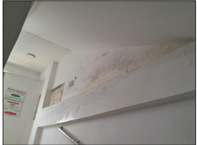
Dampness on beam
