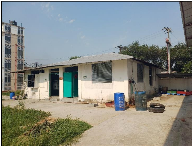
Shed:2 (Generator and sub-station)
