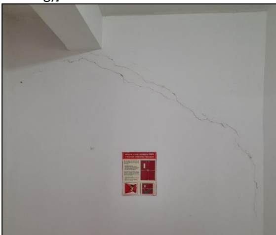
Crack on a brick wall (stair zone of 3 rd floor)
