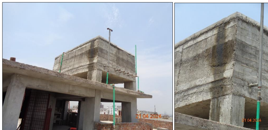
Seepage in RC wall of OHWT
