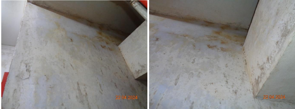
Seepage in RC wall of under-ground water reservoir
