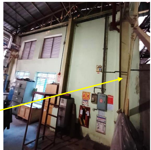
Orientation mismatch - marked columns
