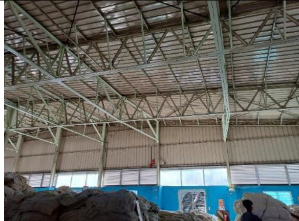
Misalignment of steel truss
