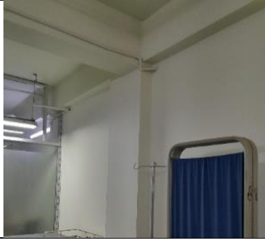
Wrong column retrofitted
