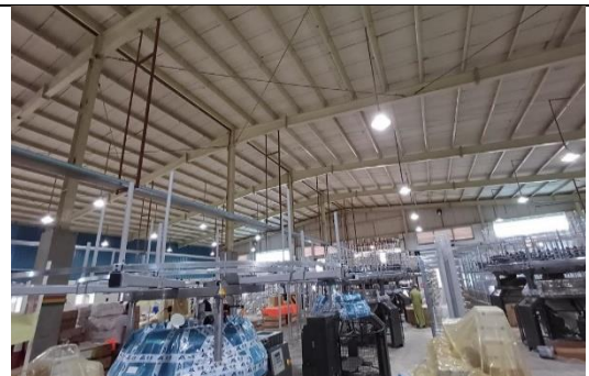
No wall bracing and rafter retrofitting
