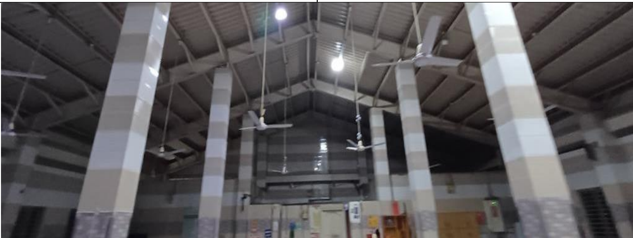
No roof or wall bracing
