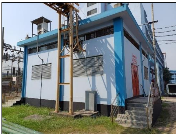
33 KV Sub-Station Room
