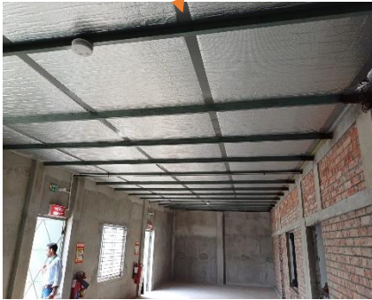
Non-engineered shed over idle machine room.
