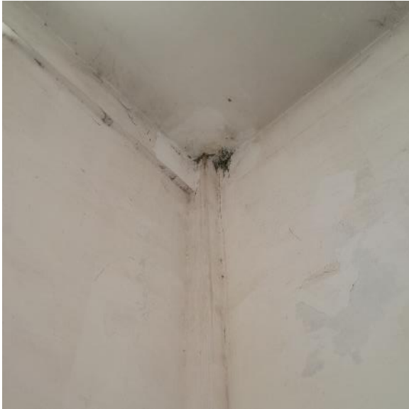
Dampness on stair roof slab
