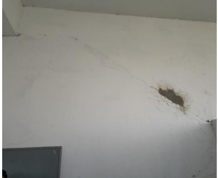
Brick wall crack at toilet zone
