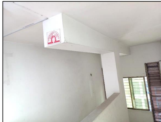
Discontinuous rooftop beam
