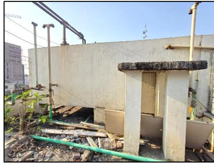
Overhead water tank at roof
