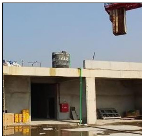
Plastic Water Tank – Not Braced
