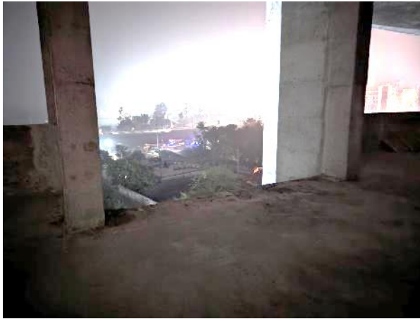
Falling Hazard on 4 th floor
