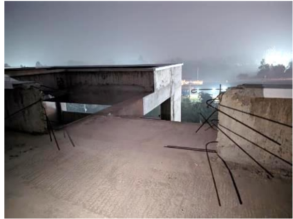
Falling Hazard on roof level
