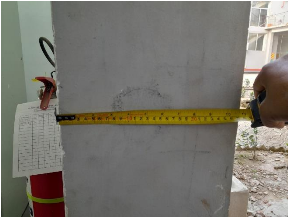
Mismatch in column dimension
