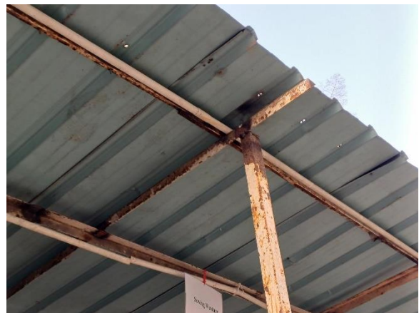
Poor steel rafter-column connection
