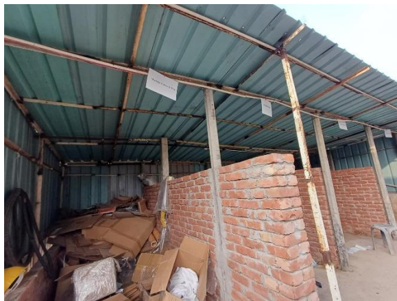
Inadequate steel members
