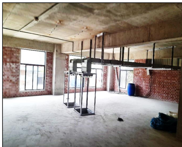
Falling Hazard on 1 st floor
