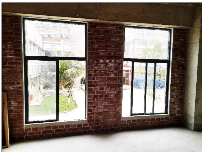
Falling Hazard on 1 st floor
