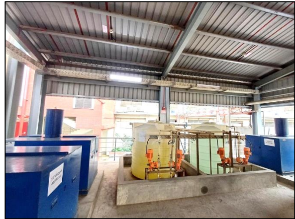
No bracing and no compression strut along eave (Shed 3)
