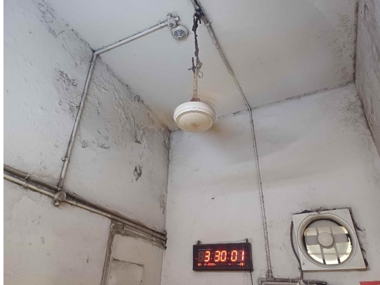
Dampness at the interior wall
