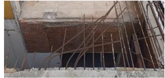
Incomplete Slab construction.
