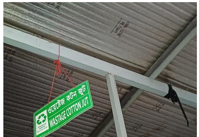
Apparently inadequate connection
