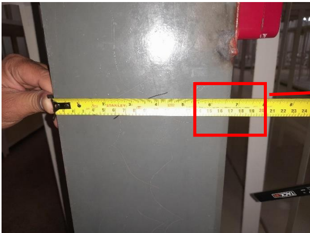
SC1 column flange measured 168 mm
