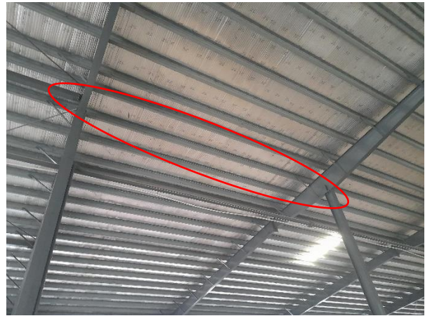
No vertical or Horizontal bracing
