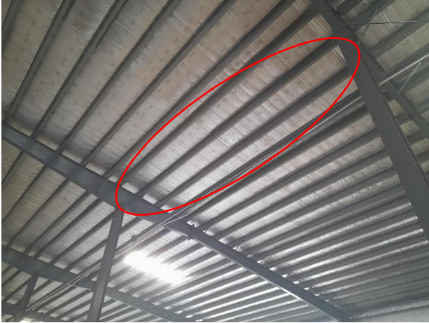
Missing compression strut
