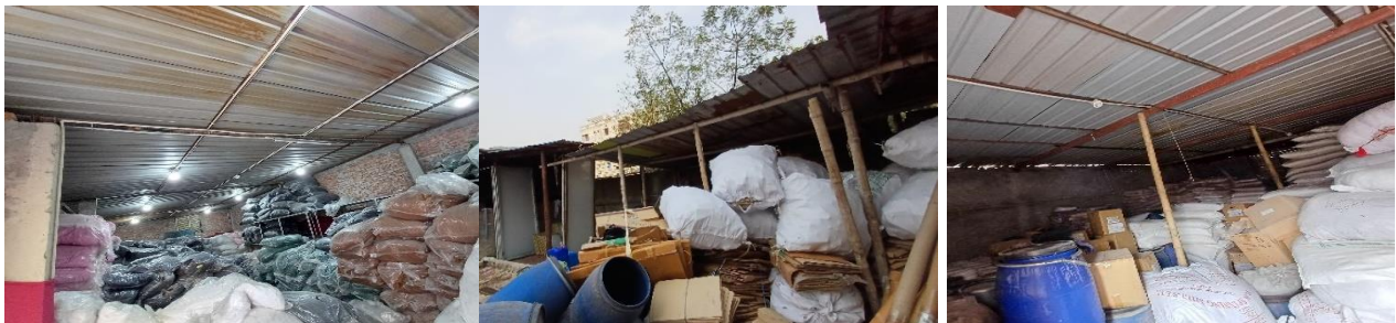
Apparently non-engineered shed: steel roof supported by RC, steel and bamboo columns
