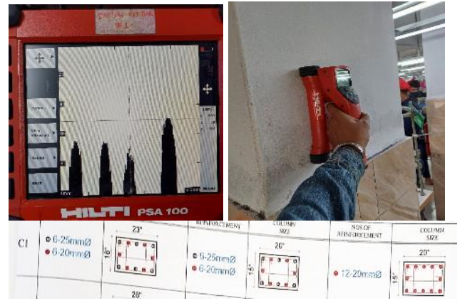
Column C1 (375X500) re-bar profile found by scanning 4/3 (10 no's) instead of 5/3 (12 no's)
