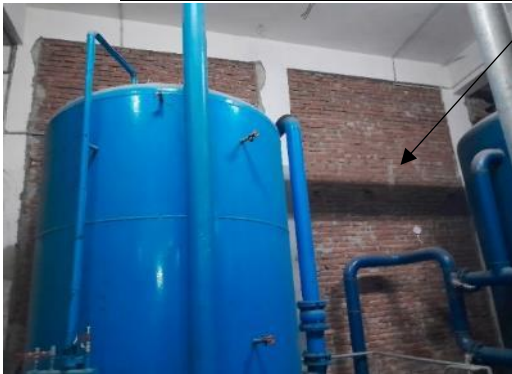
Missing share wall
