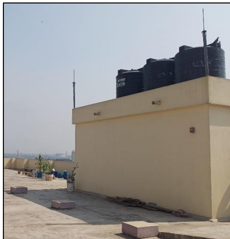
Unbraced PVC tank on the roof
