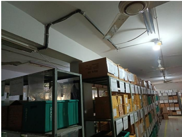
Unbraced racks on floor
