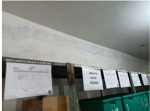
Cracks on load bearing wall
