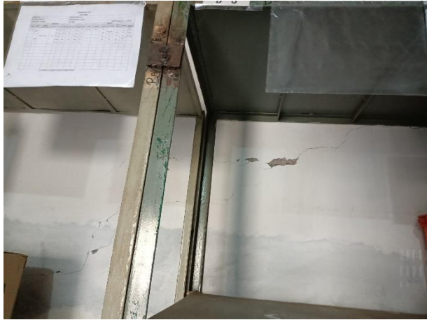
Cracks on load bearing wall
