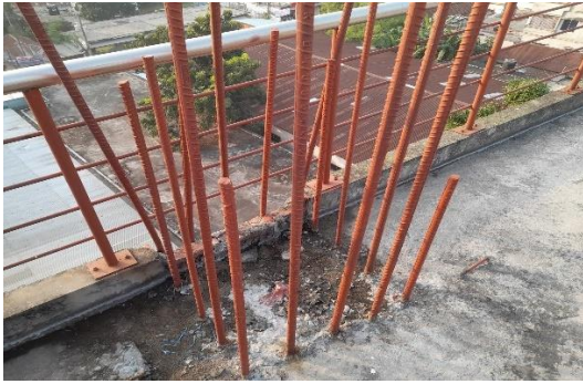
Column C2 exposed rebar at roof
