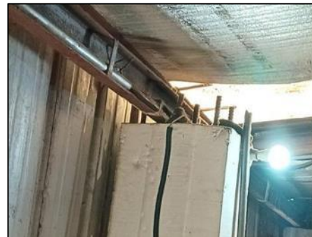
Poor connection between rafter and RC column (Kitchen Shed)
