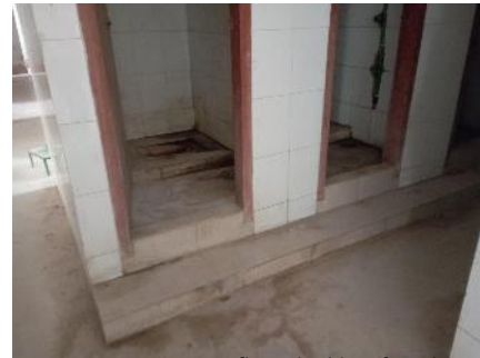
250mm floors build up found at toilet zone.
