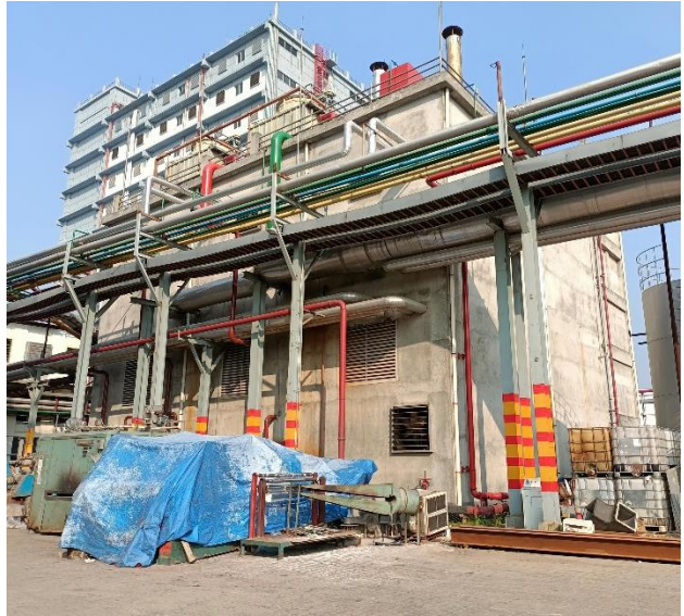
Thermic Fluid Heaters & Chiller Building
