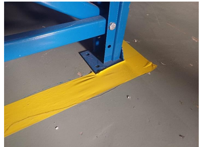
Unbraced racks on the floor
