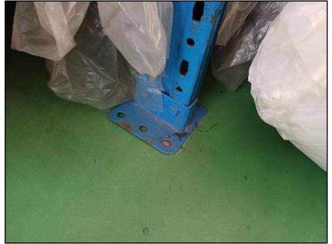
Unbraced storage racks
