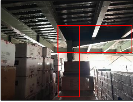
Frame section missing in the prepared drawing
