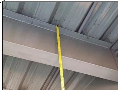
Sub beam size was found (125x350) mm instead of (100x200) mm
