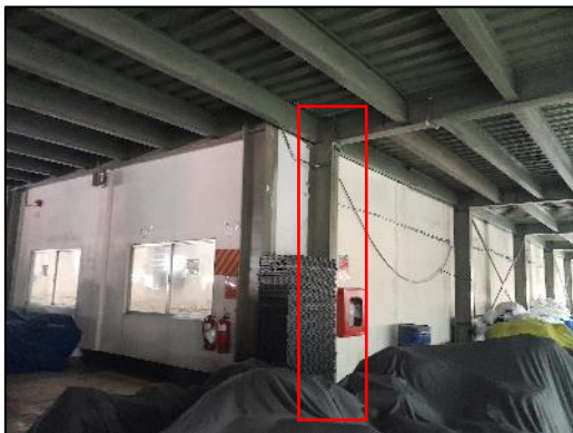
Undocumented steel column
