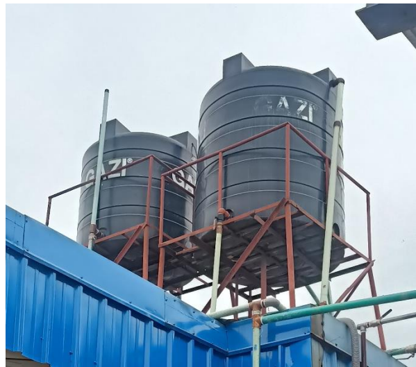
Plastic water tank on roof
