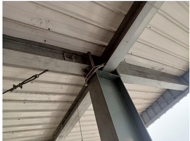
Improper bracing connection
