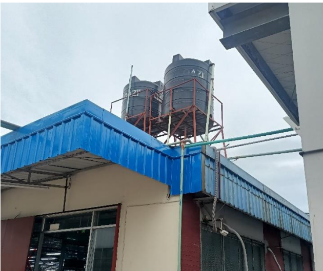
Plastic water tank on roof
