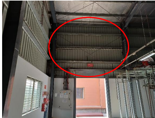
Mismatch in side wall bracing section
