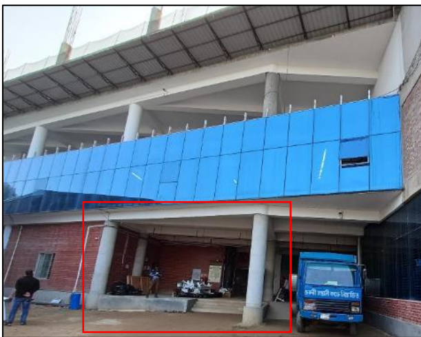
Columns susceptible to vehicle impact.
