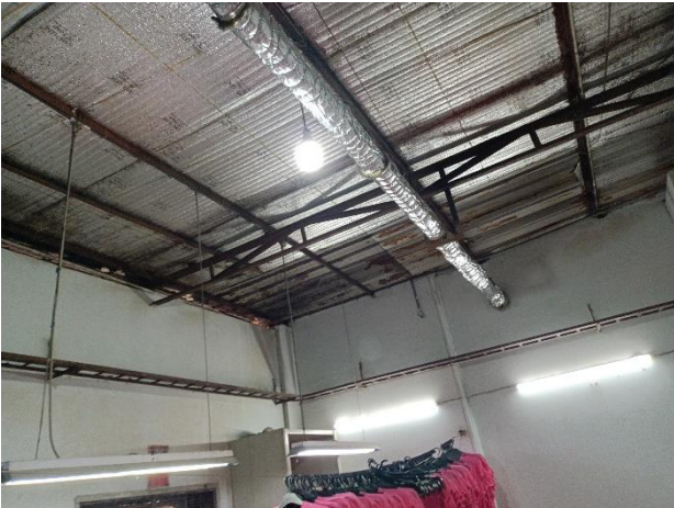
Corrossion on steel truss
