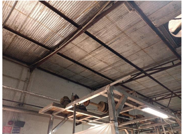
Corrossion on steel truss
